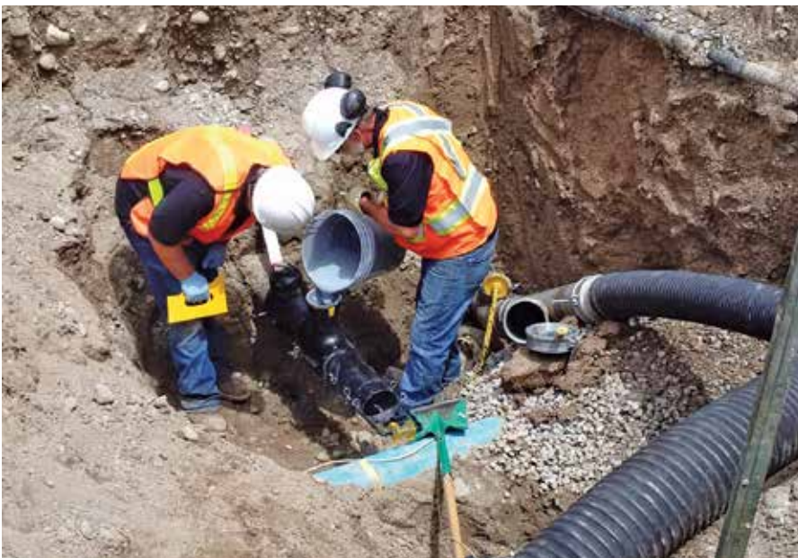
AFTER THE WATER LINE WAS CLEANED, CREWS BEGIN TO ADD THE TOMAHAWK BARRIER COATING.
