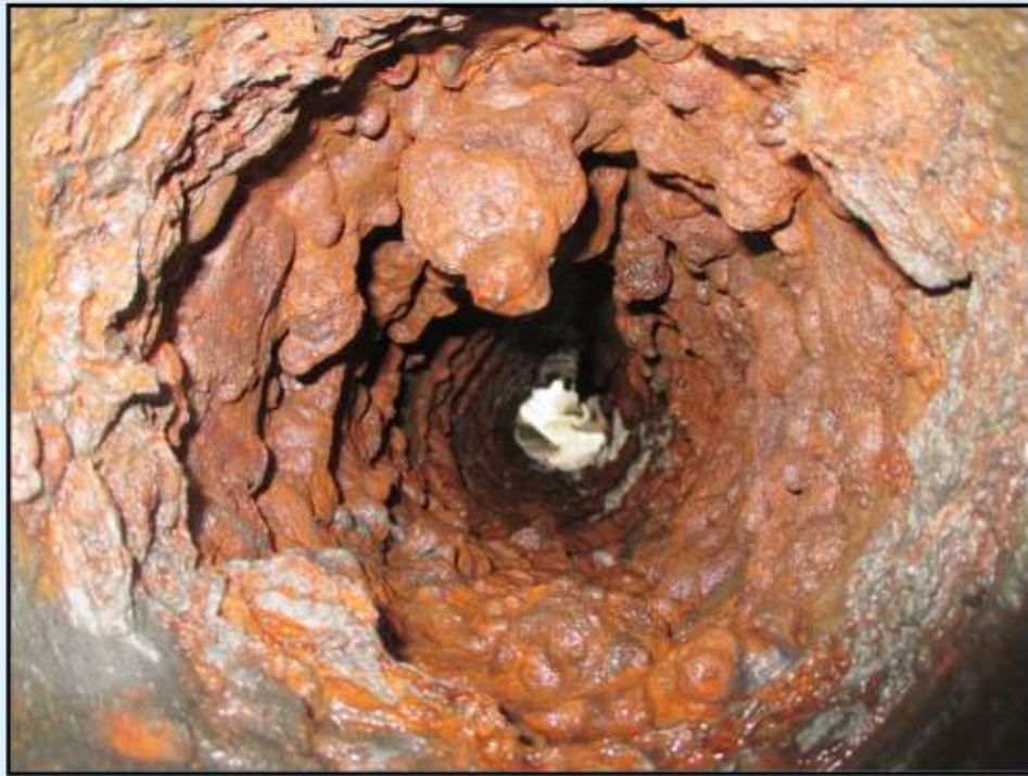
6" tuberculated water main. Photo by Envirolitics
