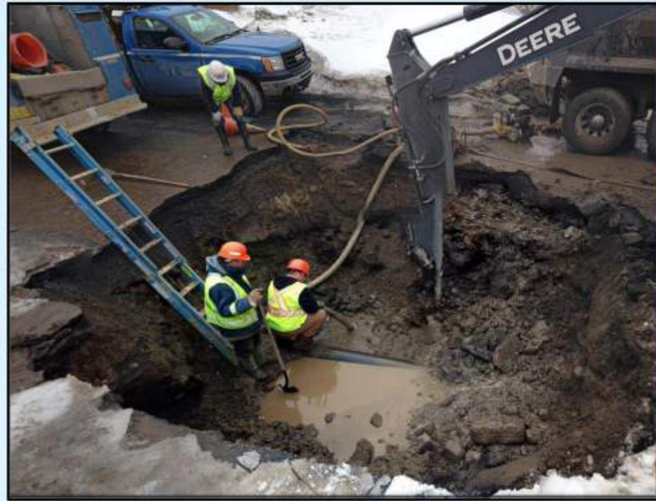
Water main break and repair. Source: Google Maps
