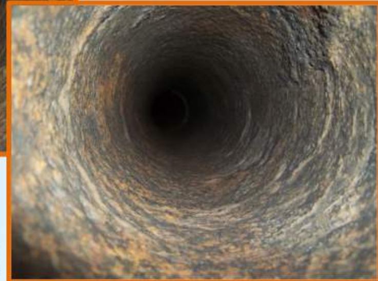
Full tuberculation removal, bitumen liner visible
