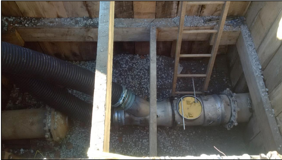
Top, single vac hose connection. Bottom, two vac truck connection for 10" and 12" cleaning
