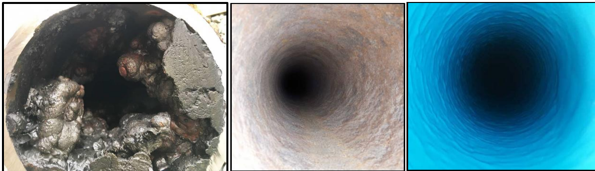
Pictures: Above left, watermain before cleaning, center, after cleaning with Tomahawk, right, after lining with Tomahawk BluKote™.
