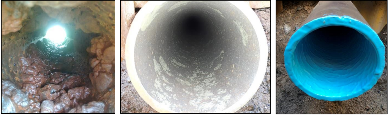
Pictures: Above left, watermain before cleaning, center, after cleaning with Tomahawk, right, after lining with Tomahawk BluKote™.
