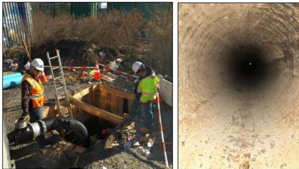
Above, Tomahawk cleaning a 12" watermain under a railway line, see rail cars in background. Above right, the clean and dry pipe ready for CIPP lining.
